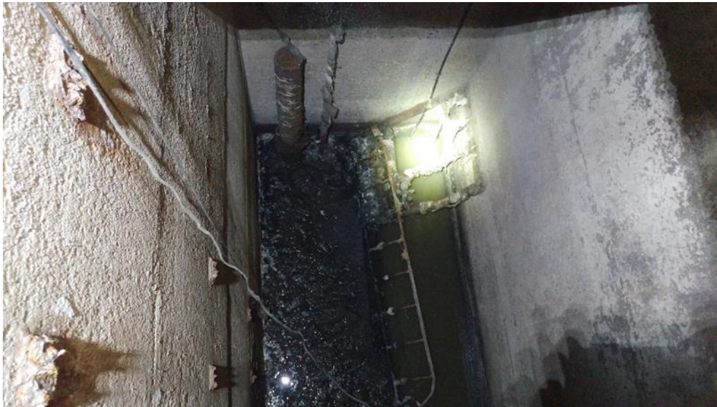
Windsor Park Wet Well
